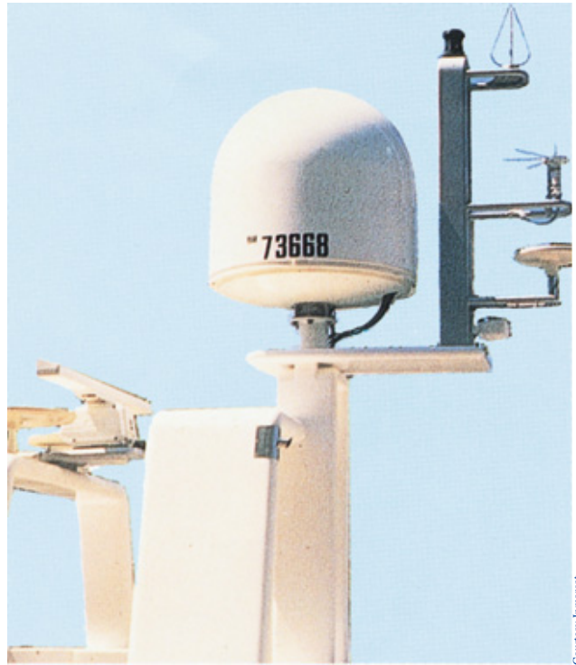
Figure 57.1 Satellite antenna ship earth station
